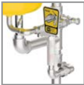
Note: Temperature sensing valve with drain back to pipe stanchion
